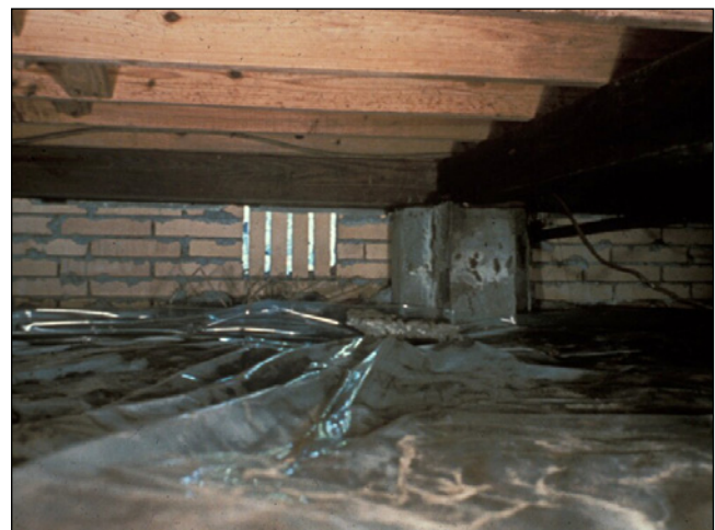
Polyethylene is widely used as a crawl space ground cover.
