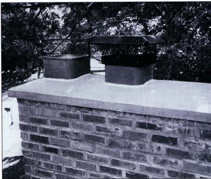
A freshly poured concrete crown is set to protect this masonry chimney for years to come.
