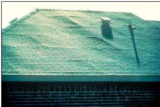
Figure 1. Outside view of failed FRT plywood roof sheathing.
