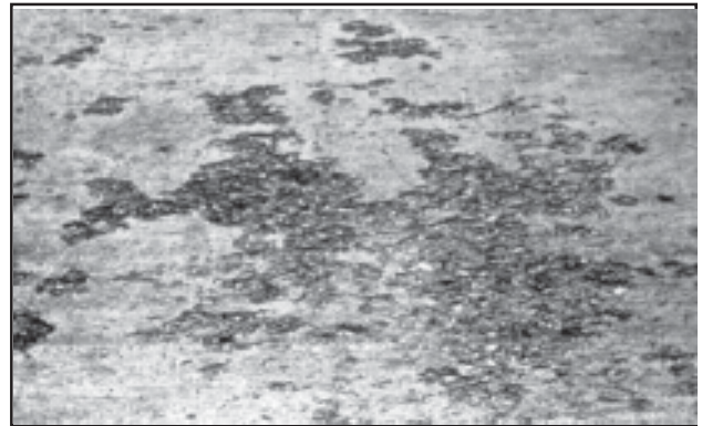
Scaling concrete surface
