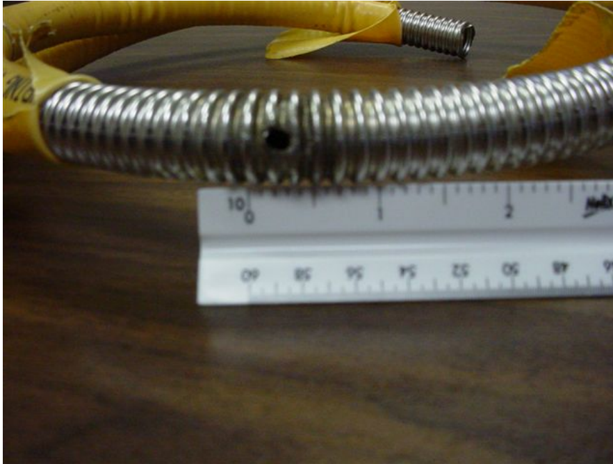
Figure 1 Typical Lightning Damage to CSST
